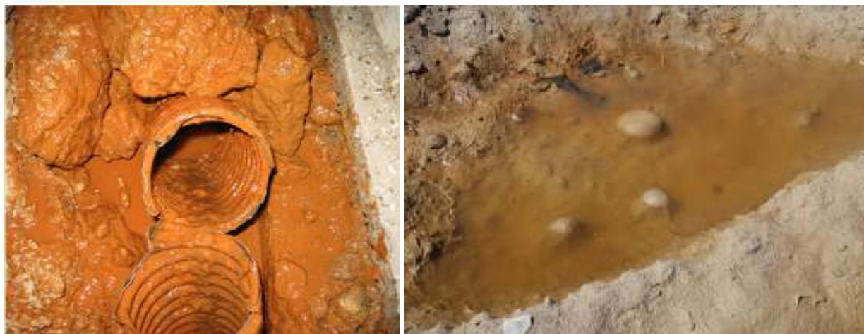
Figure 1. a. Deposits from iron bacteria plugging a drain pipe (from DiStart.com)
